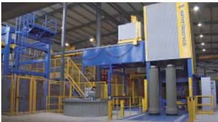
Fig. 1 The EXACT2500 production plant at a glance.
