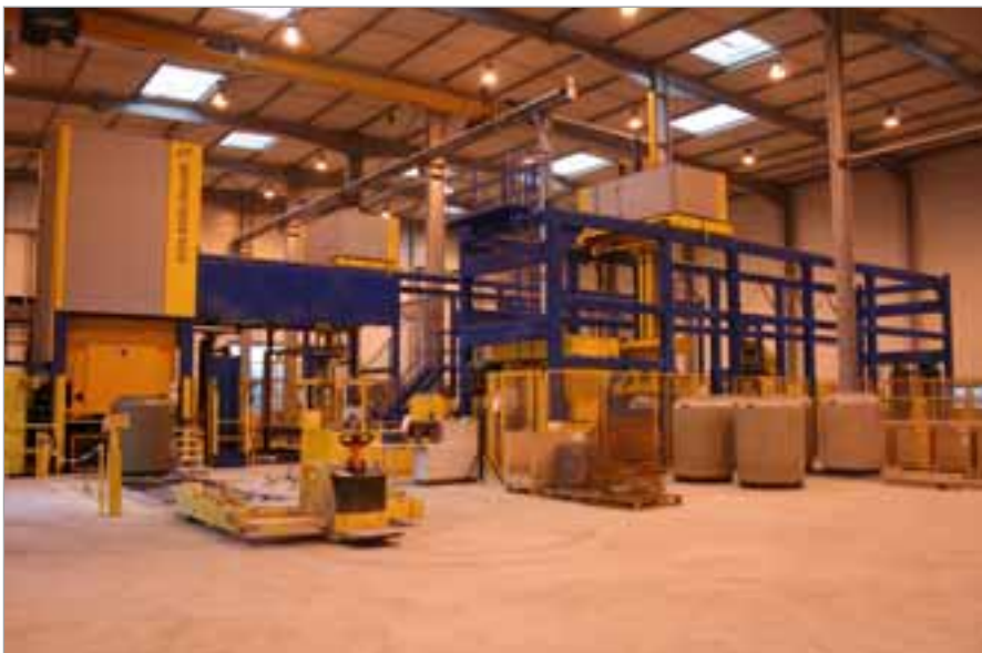
At Plattard in Villefranche, France, a brand-new Exact manhole production plant has been started up recently.
