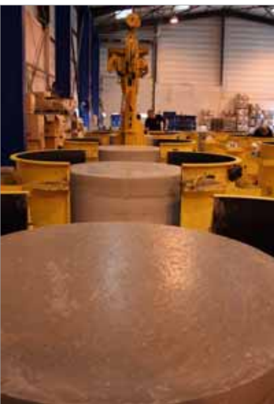
After one day the manhole bases which were produced the day before are dismantled.
