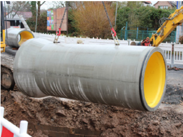
Figure 3: Inserting of a pipe in the trench by using a chain sling fixed on two anchors
