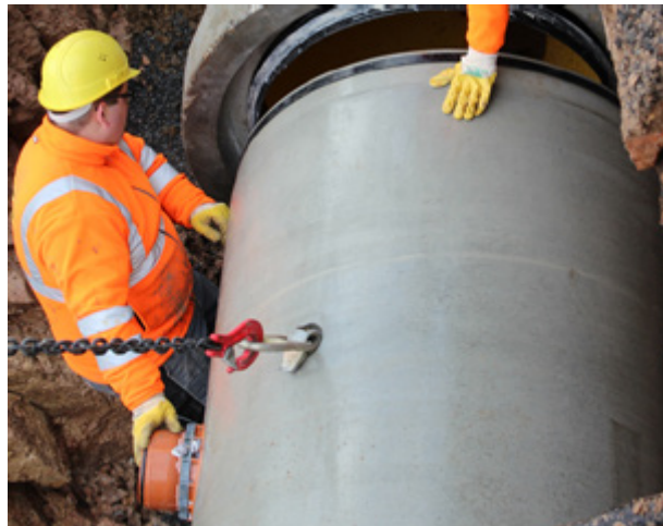
Figure 4: Connection of a reinforced Perfect Pipe DN1000 to the already installed new sewer section
