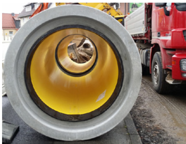
Figure 1: Reinforced concrete Perfect Pipe DN 1000 with pre-integrated connector right before installation at the building site in Sandershausen, municipality of Niestetal
