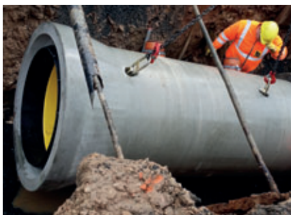
Safely setting down of a pipe into the trench before connecting to the already existing new sewer channel.
